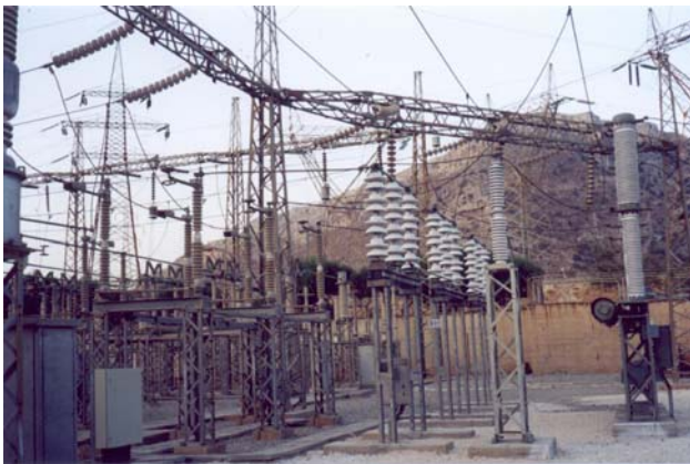
Figure 9 Coated Porcelain insulators at Linoperamata Substation
