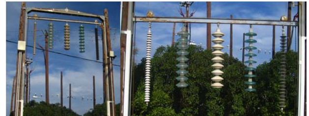
Fig. 4. Photos from the pollution measurement arch (upper and lower position of insulators)
