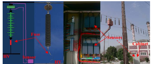
Fig. 6. A drawing of the basic leakage current measuring installation and photos from the actual installation in TALOS High Voltage Test Station
