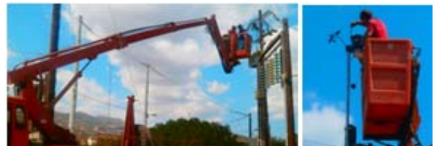
Fig. 5. Installation of the weather station on top of the pollution measurement arch
