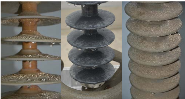
Hydrophobic class 1 Hydrophobic class 7 Hydrophobic class 1 Fig. 4: Hydrophobicity classification of field composite insulators in high voltage network of Crete according to STRI [22]
