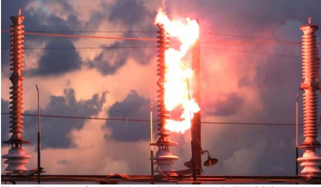
Fig. 9 : Flashover of post outdoor 150kV insulators in TALOS[39]
