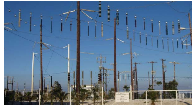
Fig. 8 : Suspension 150kV Insulators in Outdoor High Voltage Laboratory in Crete (TALOS)[39]
