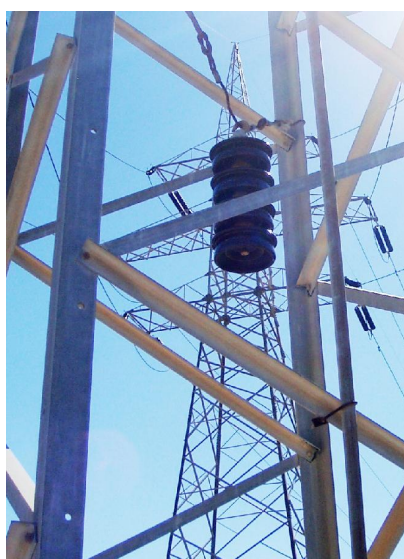
Fig. 4 A string of insulators (fog profile-porcelain) hanged (offline) from the metal structure of a 150 kV tower
