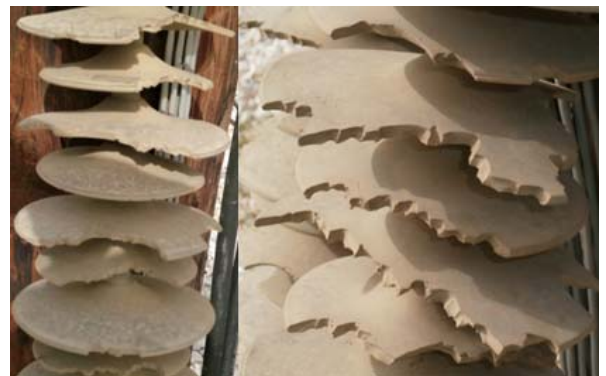
Figure 2. Polymer insulators attacked by birds
