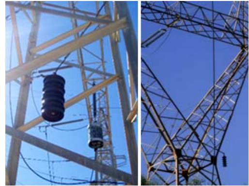
Fig. 5. Dead strings hanged from the metal structure of towers
