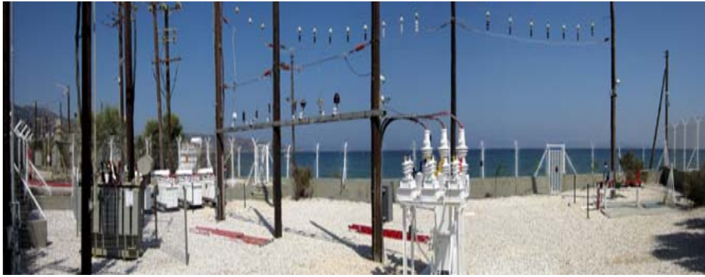
Figure 2. Photograph of the TALOS insulator test station in Iraklion Crete (21 kV bay)
