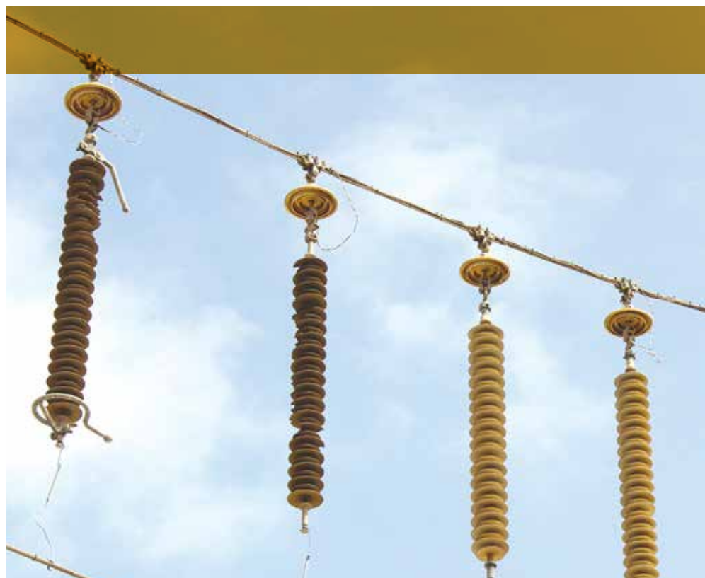
Examples of degraded insulators hung at Talos Test Station.
