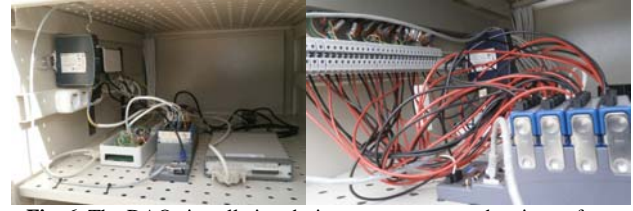
Fig. 6. The DAQs installation during a test run-up and a picture from the latest set up
